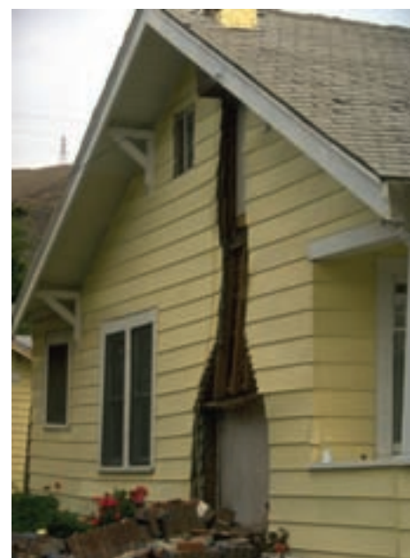
Quake damage to a residential building in Santa Monica, California.
